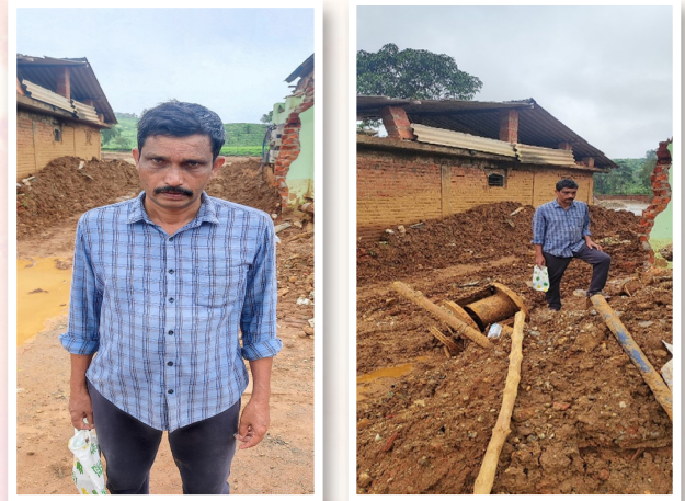
Reji with the demolished shop by the landslide
