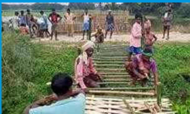
Community working together for construction of a bridge in Balwa Santhali village, Bihar
